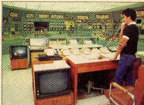
Control Room: Never to produce a watt
