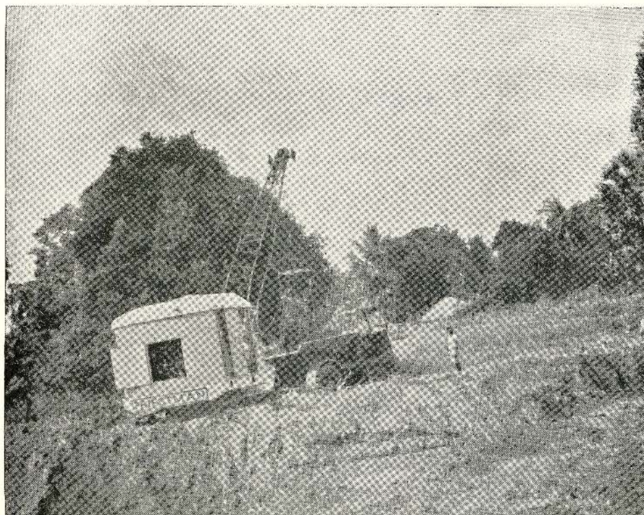
Dragline excavator, dumper and loader working as one unit on future reservoir
