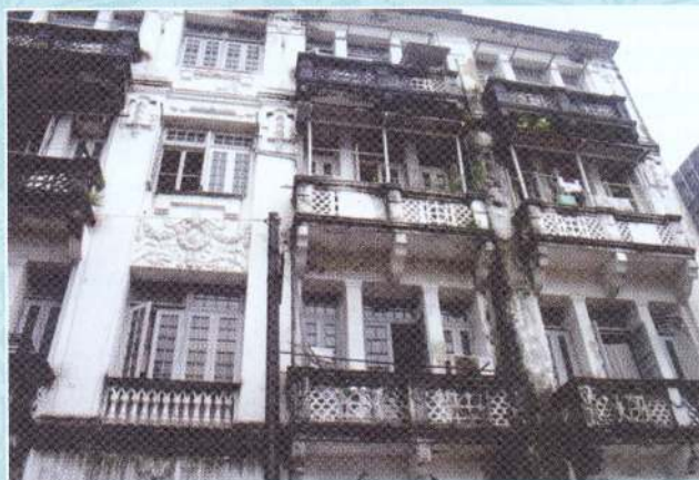
The Thamby family occupied the large flat on the top most floor. Picture was taken in 2011. This flat is more than a century old.
