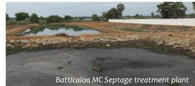
Fecal sludge unloading point
