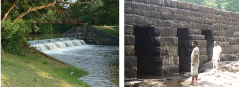
Inlet Thekkam anicut to diversion canal to Giants Tank and Downstream view of Thekkam anicut in Mannar
