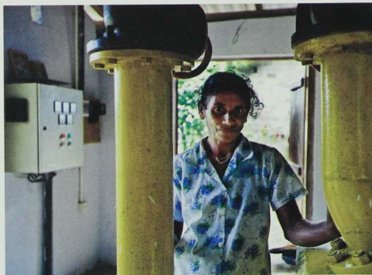
Y. G. Chandrawathi manages the power house of a Micro-hydro project. Renewable Energy for Rural Economic Development Project.
