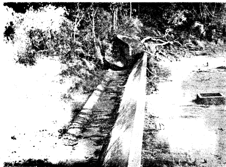
35.2 KOTIYAGALA MAHA WEWA—SPILL
