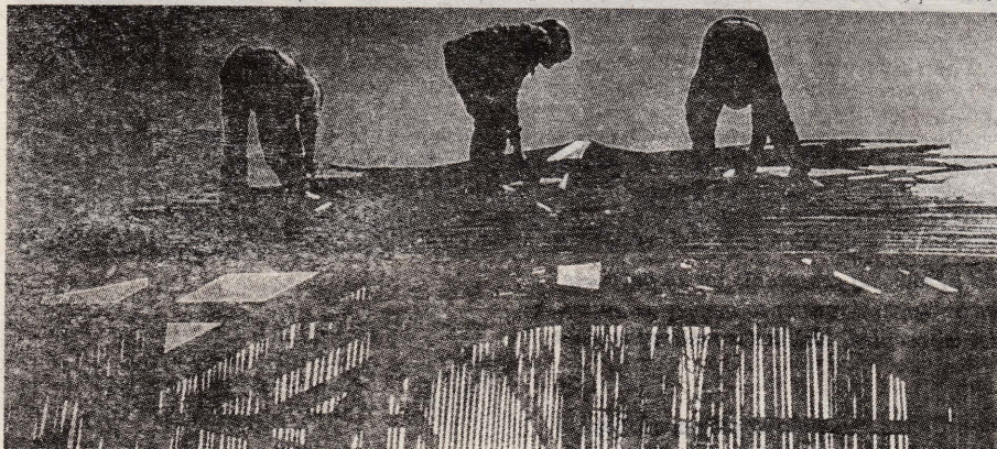
SHELTER HELPERS: Residents construct a building out of straw. Almost all the housing in Villa El Salvador is built by community volunteers.
