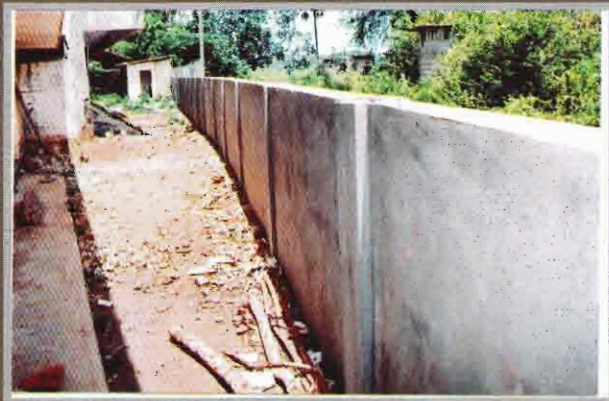
Western side new boundary wall behind Jeyaratnam block supported by the Foundation
