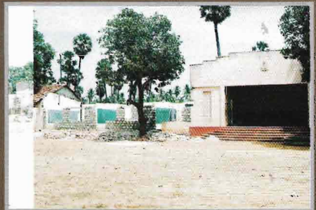
3 classrooms between A/L block and open stage being renovated - work in progress
