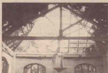
War Damaged St. Johns Staff room
