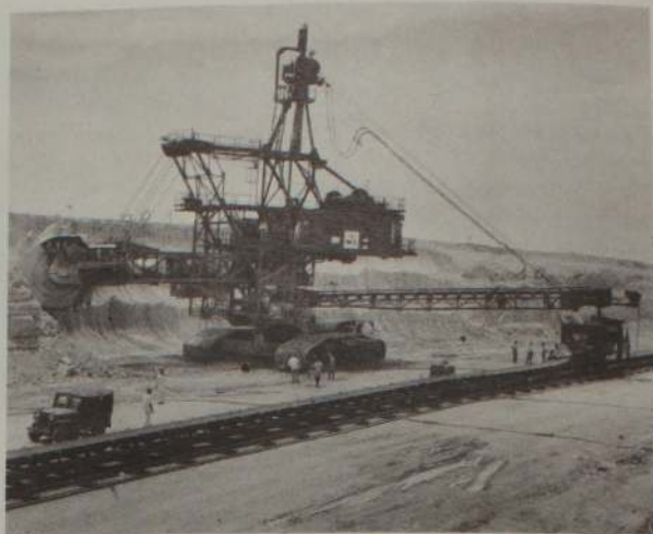
Bucket wheel excavator at the Nyveli Lignite Project, Madras, India, assisted by the United Kingdom and the United States.
