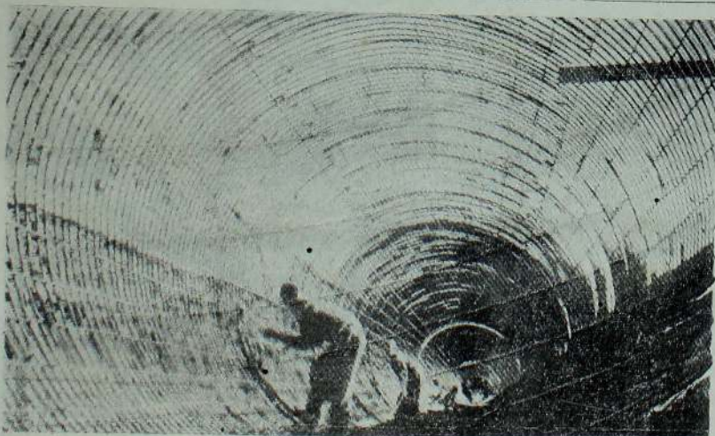
In pix Ingra's technicians are seen placing reinforced steel bars in the tunnel presently been constructed in Zambia.
