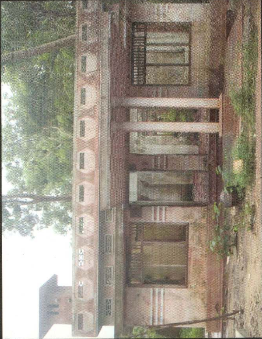
A damaged house
