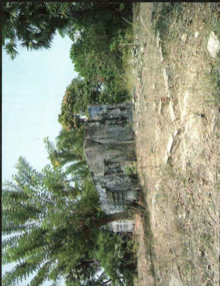
A damaged house
