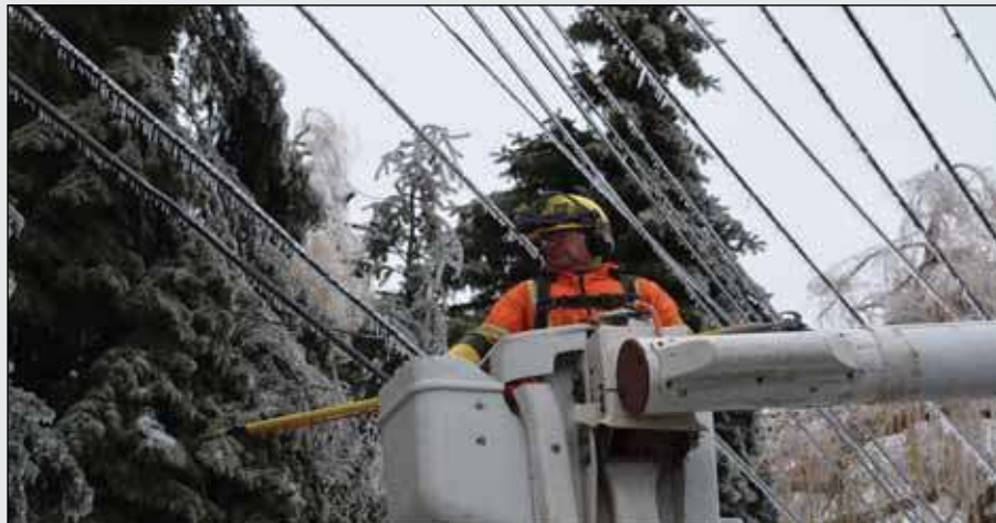
Forester, David Knight, works high above the ground to remove tree branches from overhead wires on Islington, December 23, 2103-Pic: facebook.com/TorontoHydro
