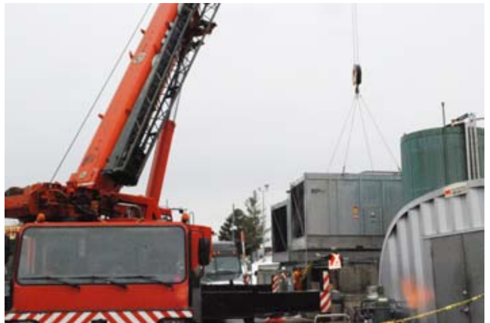
A new chiller installed last month at the General campus of TSH will help reduce cooling costs by up to 20 per cent.
