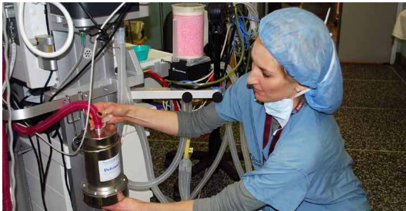
Dr. Carly Peterson, TSH Anesthesiologist, adjusts the Deltasorb canister which works in line with the anesthetic gas scavenging system to capture unused anesthetic gas and prevent venting to the atmosphere.
