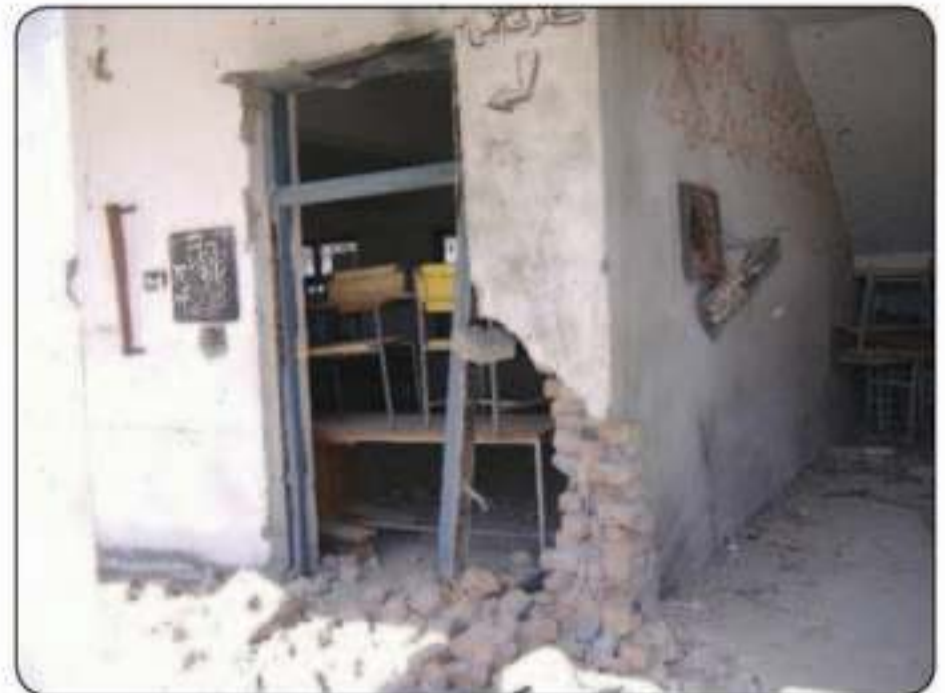
Many schools have been damaged and need to be restored – pic: Ibrash Pasha/IRIN
