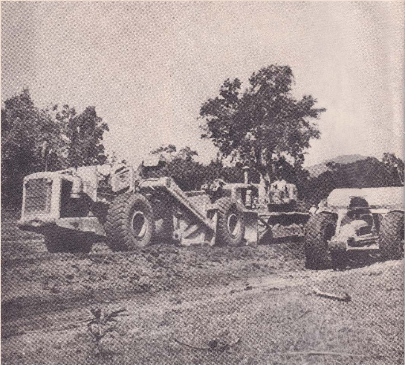
Modern U.S. road equipment was used to build a 22-mile highway connecting Aluthnuwara and Padiyatalawa.
