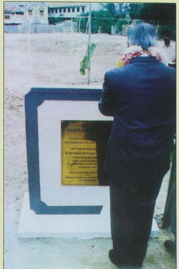
His Lordship Sarath N. Silva P.C., Unveils the Plaque after laying the foundation stone for the Jaffna Courts Complex.
